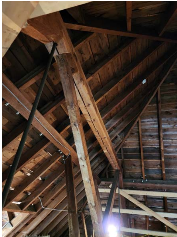
Photograph #28 (Town Hall) – Cracked Truss Member
