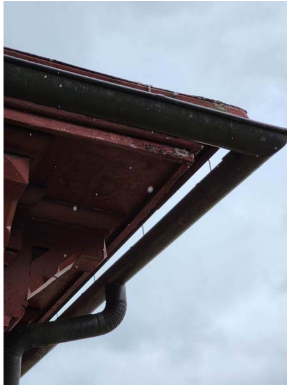
Photograph #19 (Town Hall) – Rotted Wood Trim
