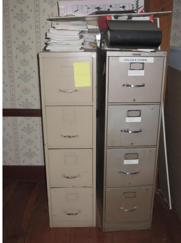
Photograph # 10 – “Storage 1” Sloped Floor
