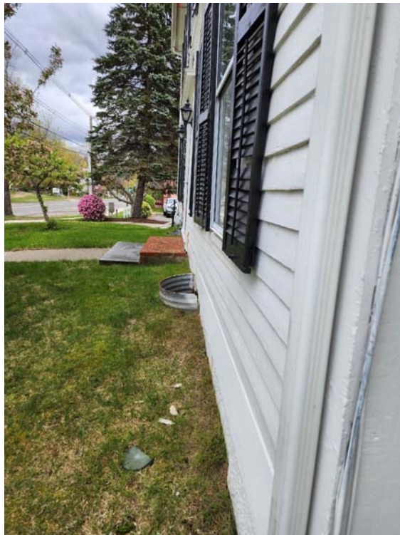
Photograph #10 (Town Hall Annex) – Bowed & Leaning Front Wall
