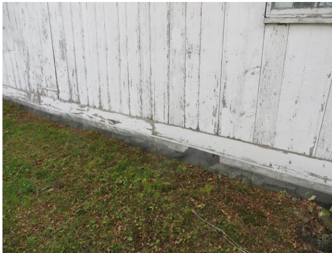
Photograph #22 – Missing “Storage” Foundation
