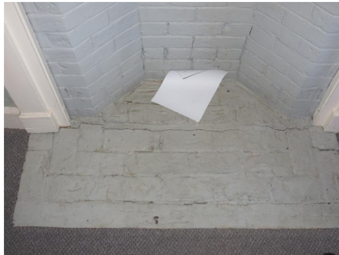
Photograph #13 – “Conservation” Cracked Masonry Hearth
