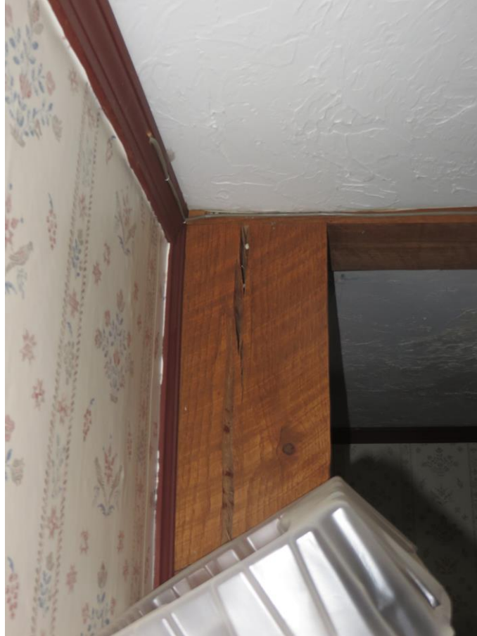
Photograph #10.2 – “Storage 1” Cracked Wood Column
