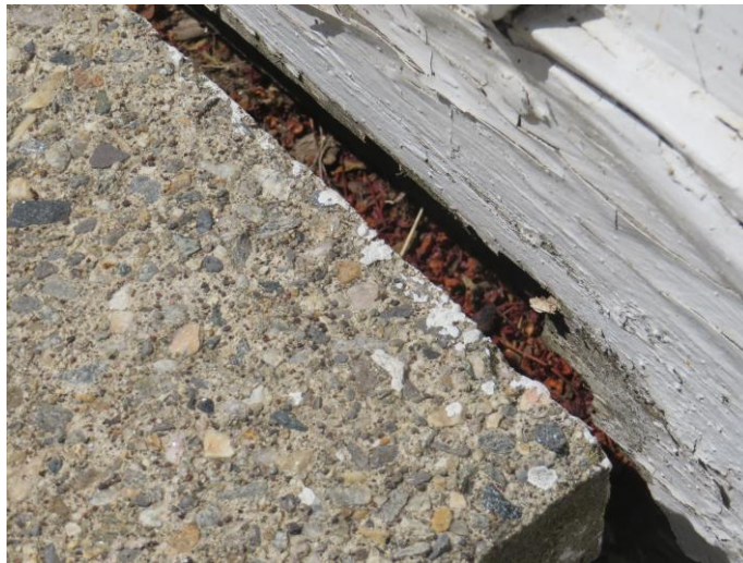
Photograph #14.1 – Rotted Sill at “Meeting” Exterior Door
