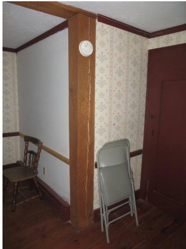
Photograph #10.1 – “Storage 1” Cracked Wood Column
