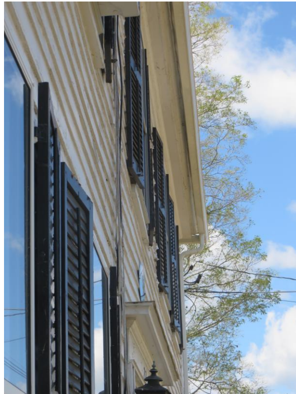
Photograph #25 – Bowed Front Exterior Wall
