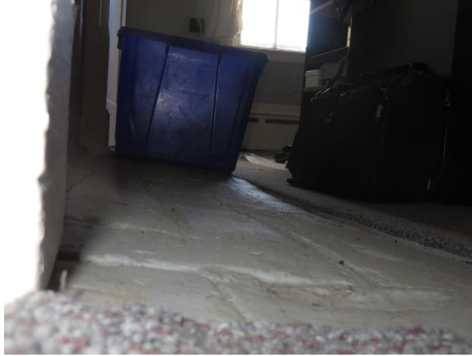
Photograph #12 – “Conservation” Sloped Floor
