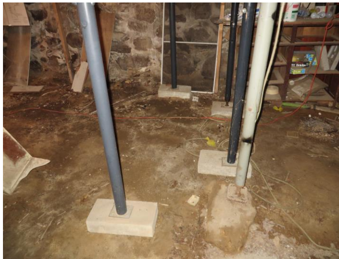
Photograph #19 – First Floor Shoring Jacks
