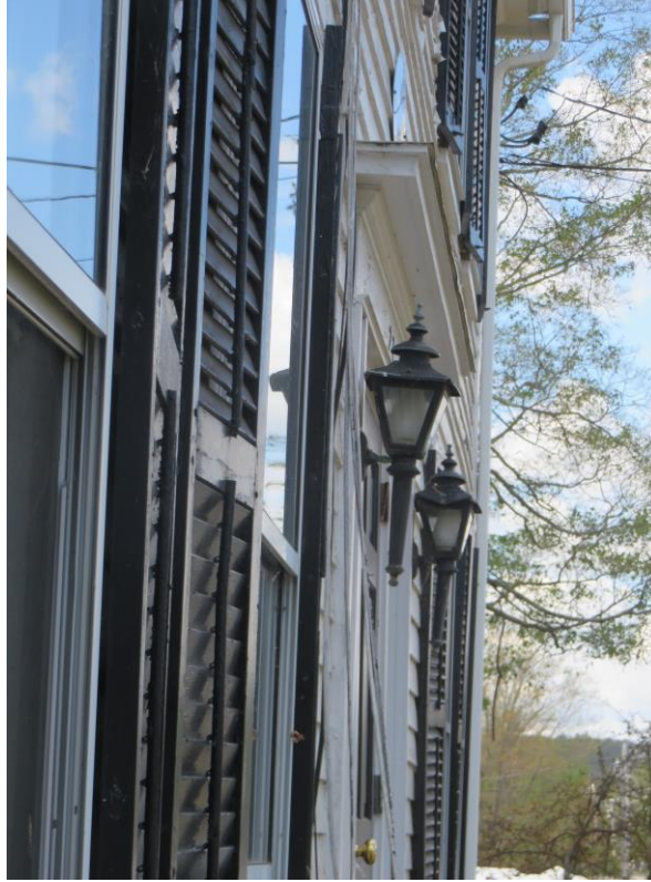
Photograph #24 – Bowed Front Exterior Wall
