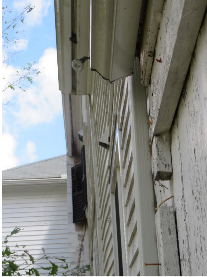
Photograph #6.1 – Exterior Bowed Wall at “Storage 1”
