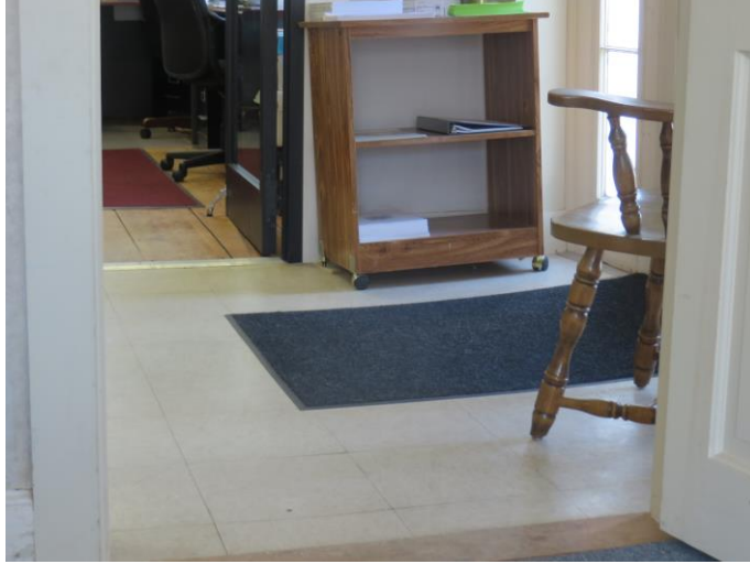
Photograph #15 – First Floor Hallway Slope
