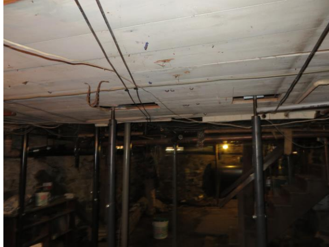
Photograph #18.1 – First Floor Shoring Jacks
