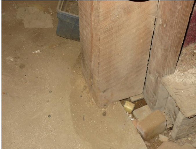
Photograph #21 -Cracked Wood Column and Concrete Slab
