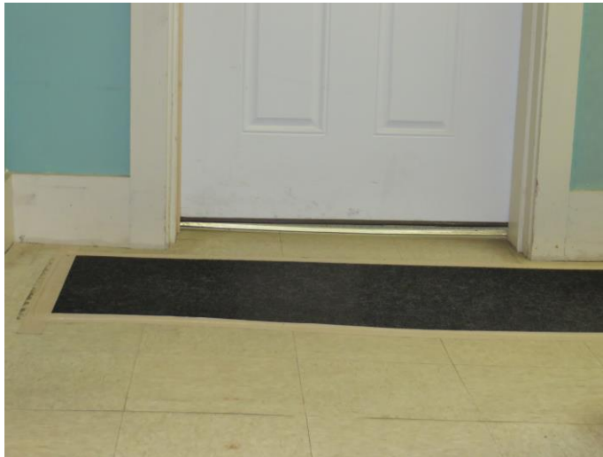
Photograph #16 – Sloped Hallway in front of Assessor's Office
