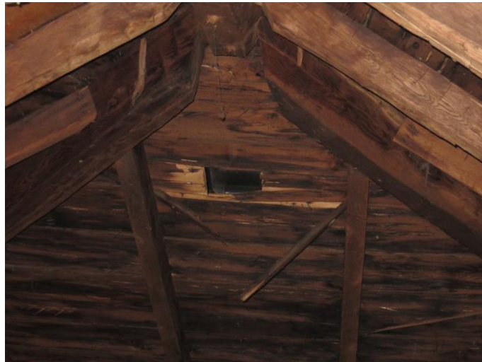
Photograph #2 – Cracked Roof Sheathing
