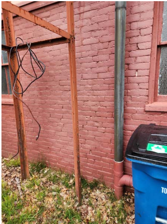
Photograph #22 (Town Hall) – Deteriorated Exterior Masonry Joints
