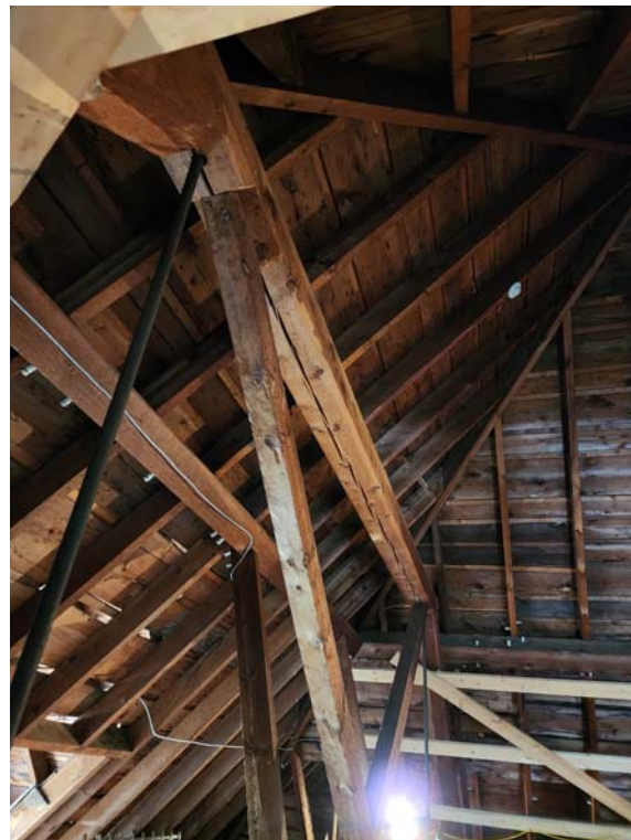
Photograph #28 (Town Hall) – Cracked Truss Member
