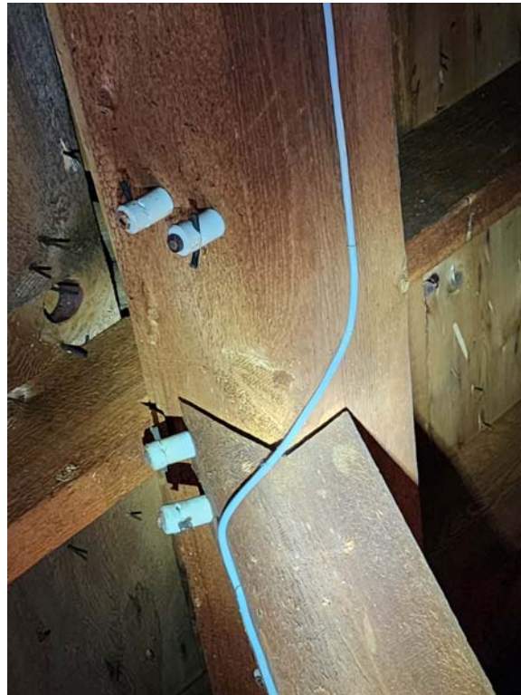
Photograph #32 (Town Hall) – Gaps at Truss Member Joint
