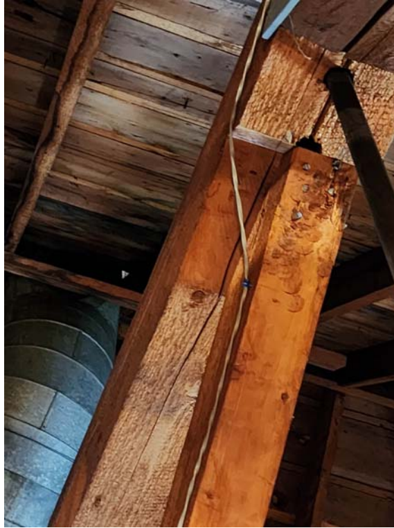
Photograph #25 (Town Hall) – Cracked Truss Member
