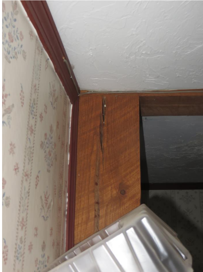
Photograph #10.2 – “Storage 1” Cracked Wood Column
