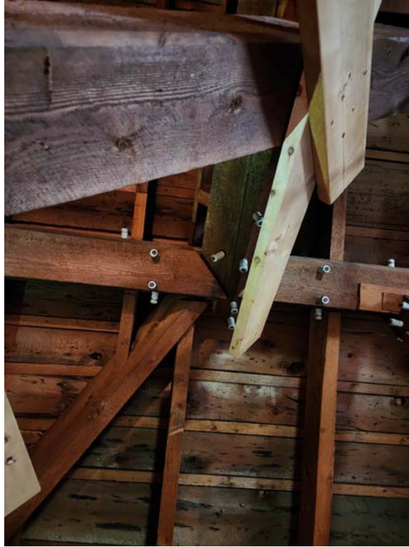
Photograph #29 (Town Hall) – Gaps at Truss Member Joint
