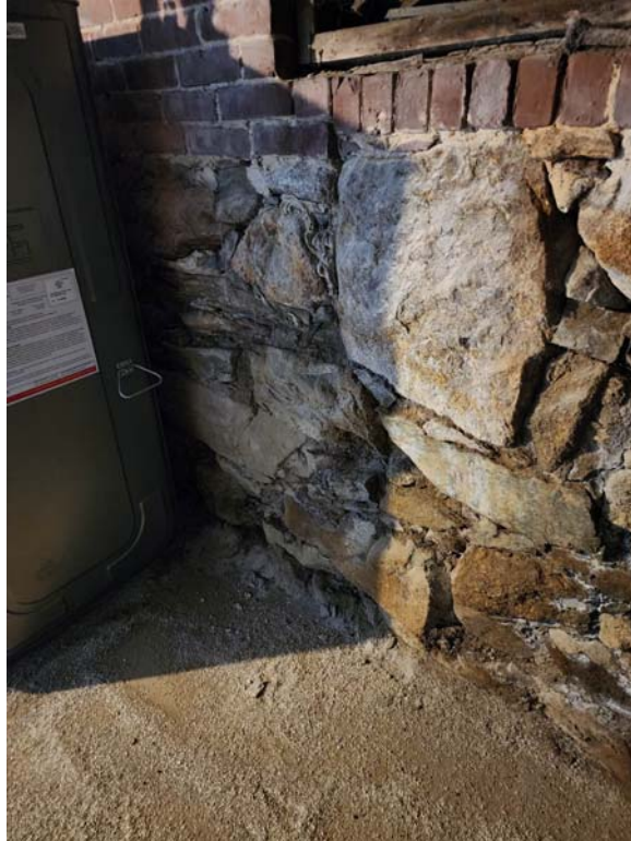
Photograph #15 (Town Hall) – Deteriorated Masonry/Field Stone Mortar Joints
