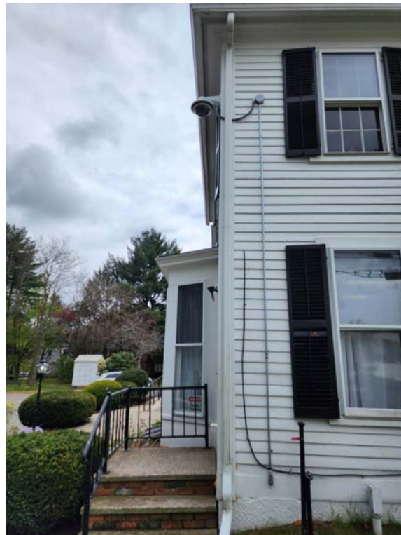
Photograph #12 (Town Hall Annex) – Leaning Side Wall
