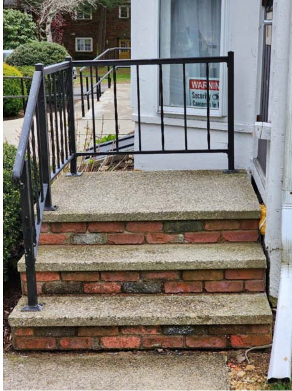
Photograph #13 (Town Hall Annex) – Sloped Exterior Side Stairs
