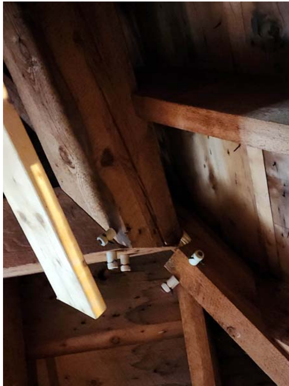
Photograph #30 (Town Hall) – Gaps at Truss Member Joint
