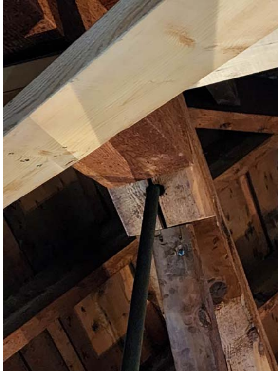
Photograph #33 (Town Hall) – Gaps at Truss Member Joint
