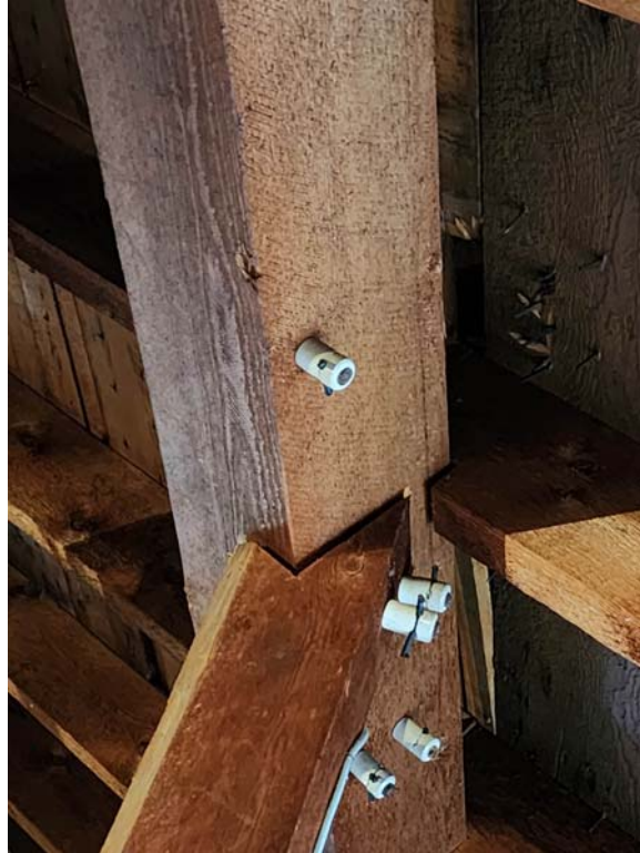
Photograph #31 (Town Hall) – Gaps at Truss Member Joint
