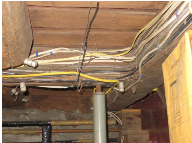
Photograph #18 – First Floor Framing (Cracked)
