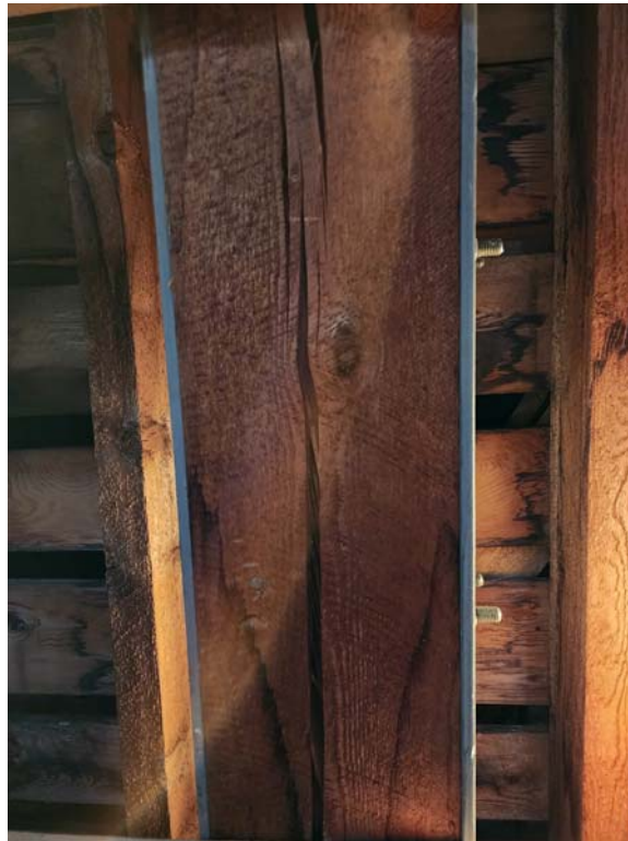
Photograph #26 (Town Hall) – Cracked Truss Member
