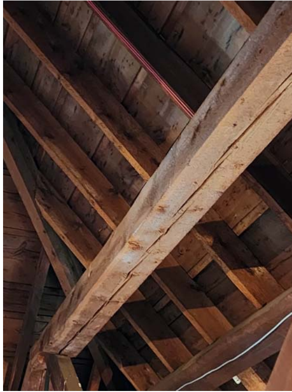
Photograph #27 (Town Hall) – Cracked Truss Member
