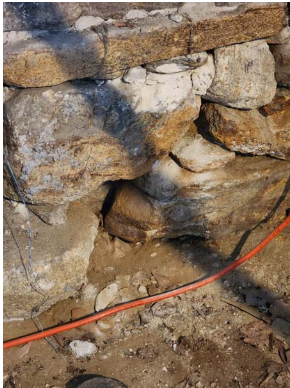
Photograph #16 (Town Hall) – Deteriorated Masonry/Field Stone Mortar Joints
