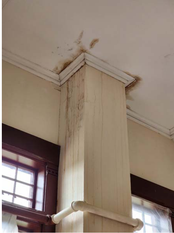
Photograph #17 (Town Hall) – Interior Water Damage
