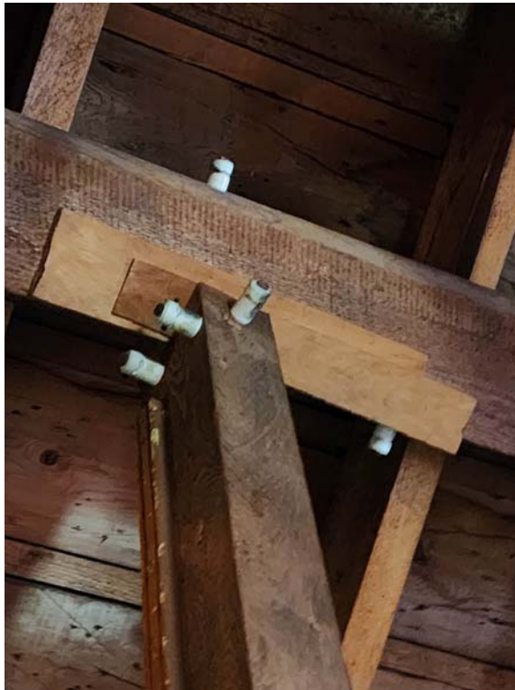
Photograph #34 (Town Hall) – Wood Shims at Truss Member Joint
