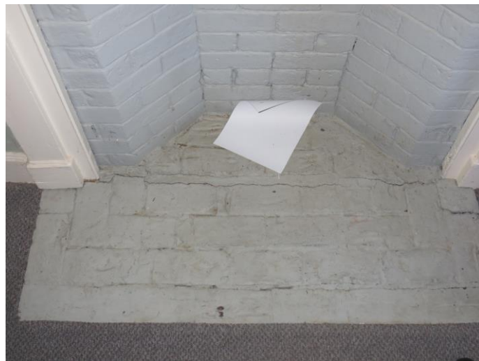
Photograph #13 – “Conservation” Cracked Masonry Hearth
