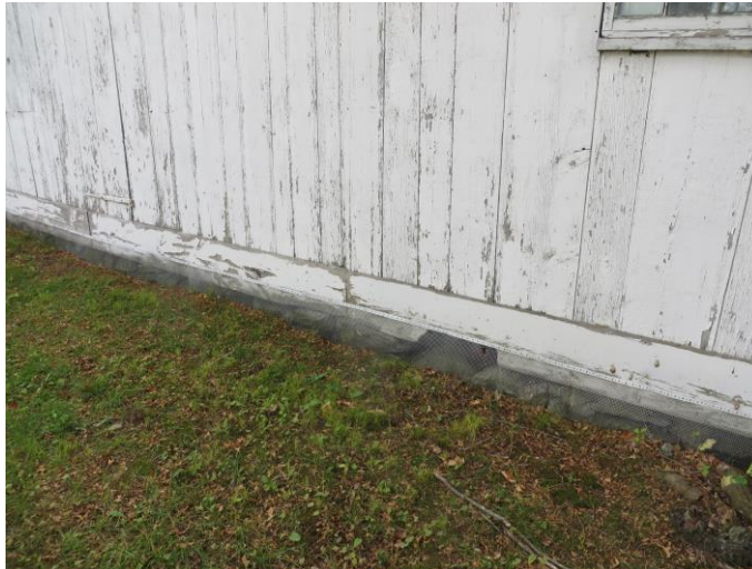
Photograph #22 – Missing “Storage” Foundation
