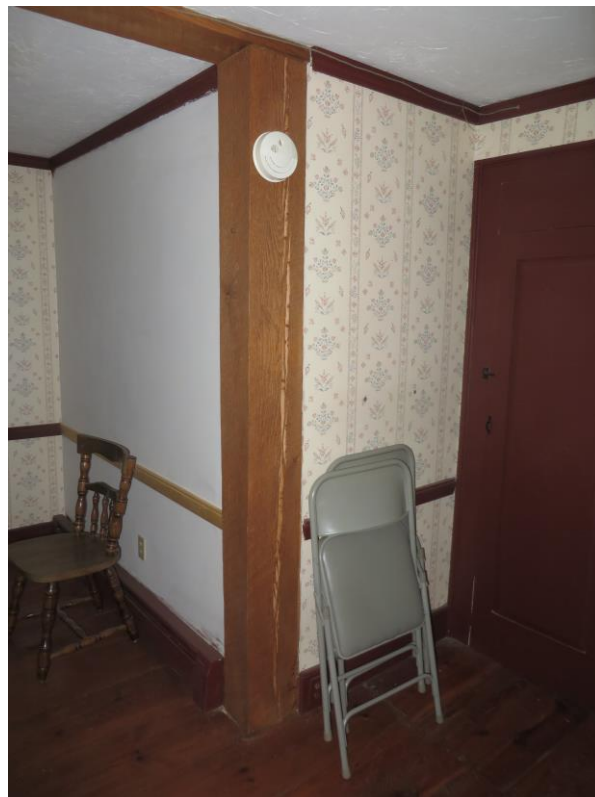
Photograph #10.1 – “Storage 1” Cracked Wood Column
