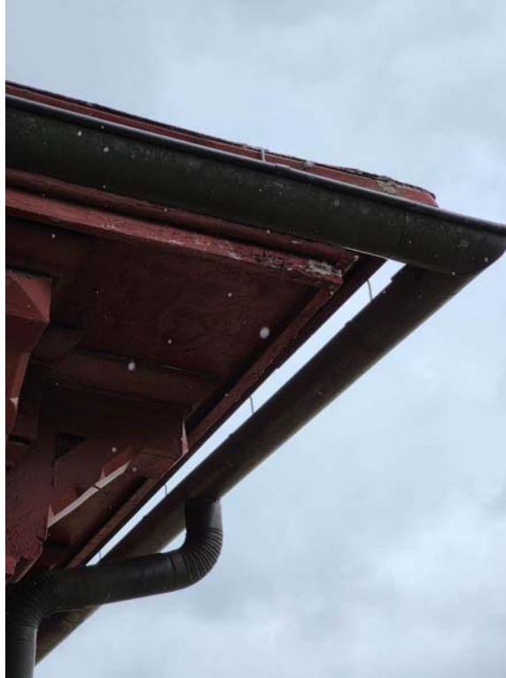
Photograph #19 (Town Hall) – Rotted Wood Trim
